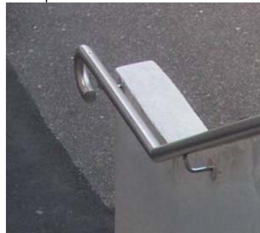
Figure 6.6: Rail extends beyond the stair.
