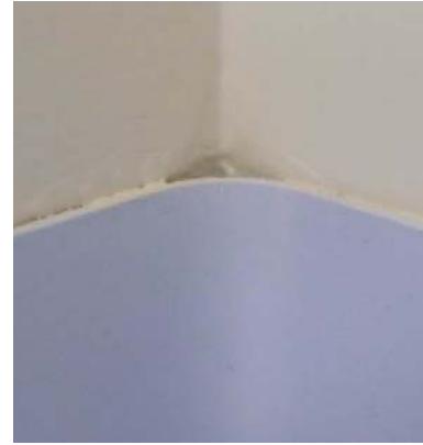
Gap between skirting and walls
