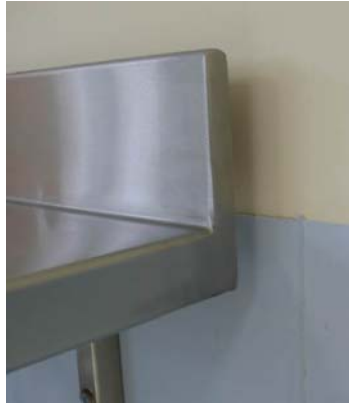
Gap between bench fitting and wall
