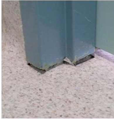
Figure 24: Gaps between door frame and floor
