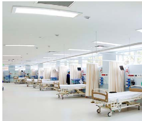
Monolithic ceilings in Stage 1 recovery areas
