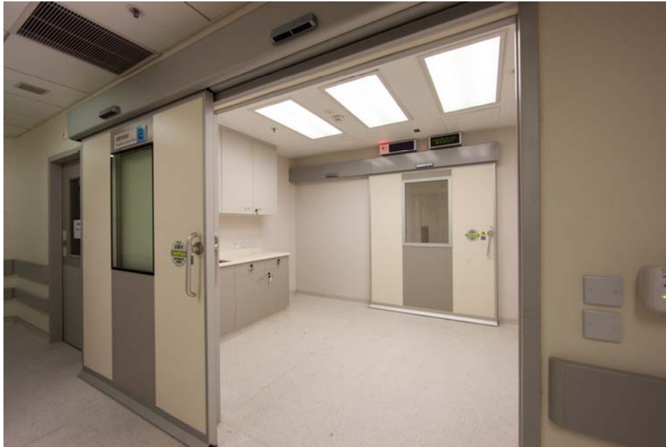
Figure 5.10: Surface mounted automatic sliding doors to Anaesthetic and Operating Rooms
