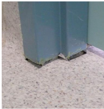
Figure 28: Gaps between door frame and floor
