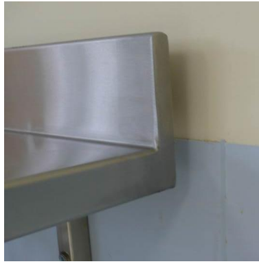
Gap between bench fitting and wall
