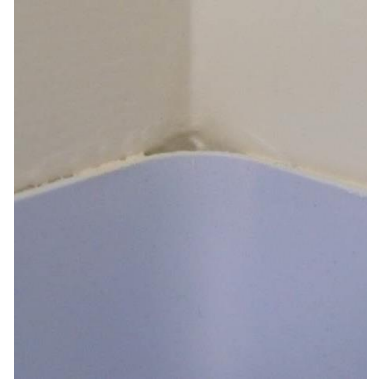
Gap between skirting and walls
